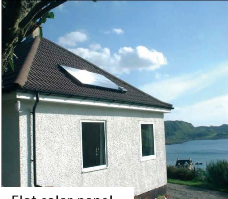
Flat solar panel
